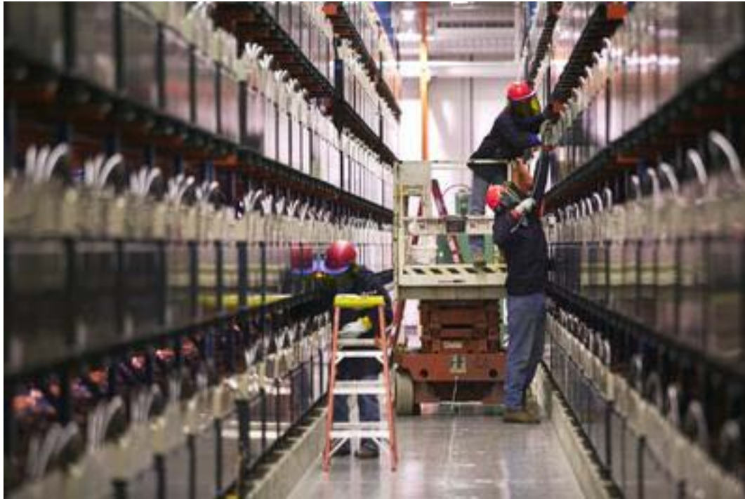
The worlds largest battery installation; 13,760 Ni-Cad cells, 5,000V 27MW/15min 46MW/5min
